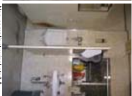
Non-compliant urinal stall & lavatory
