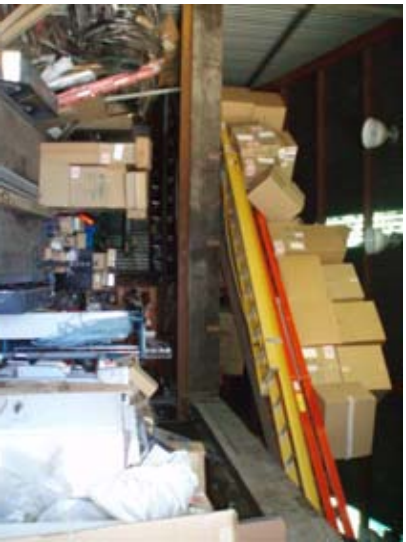
Figure 11 – Boxes are stored on a ladder placed horizontally. These constitute a falling hazard, and the storage arrangement does not meet ASCE 31 requirements.
