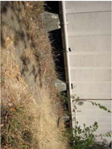
Figure 3 – The wood frame building is supported on one foot high precast concrete piers. These do not provide resistance to lateral forces.
