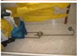
Non-compliant emergency shower
