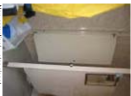
Non-compliant water closet
