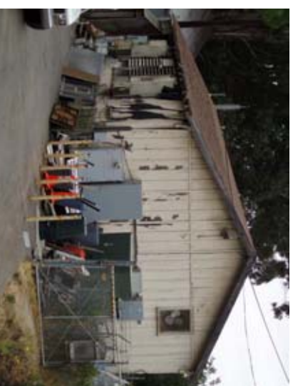
Figure 2 – Wood frame building. This is showing deterioration on its the exterior. The ends of many roof rafters are rotten and the paint is peeling off the siding in many places.
