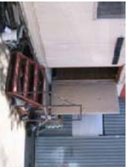
Bldg C - Stairs to office/breakroom are non-compliant
