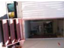
Bldg C - Stairs to toilet room are non-compliant
