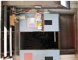
Building A - Workshop has non-compliant entry
