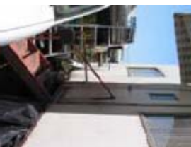
Bldg D - Stairs to small trailer office are non-compliant
