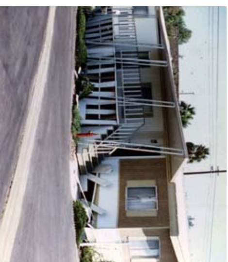
Figure 8 – An example of a trailer (mobile home) that has fallen off its supports.
